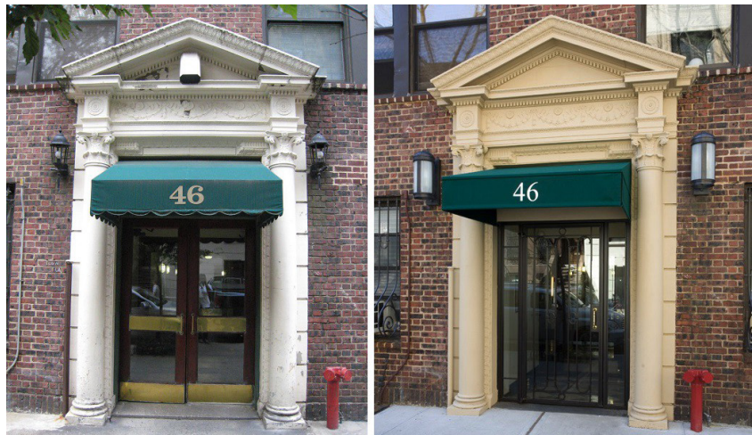
Before and after of a facade repair and door replacement for a 1923 Landmark District building. ▶
